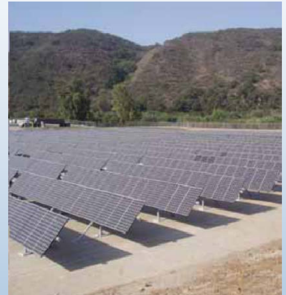
Source: SunPower – Thousand Oaks, CA water treatment plant
