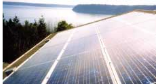
5 KILOWATT GRID-TIED PV SYSTEM
